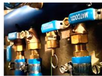
RELIEF VALVE LOCATED UNDER AER-FLOW MANIFOLD
